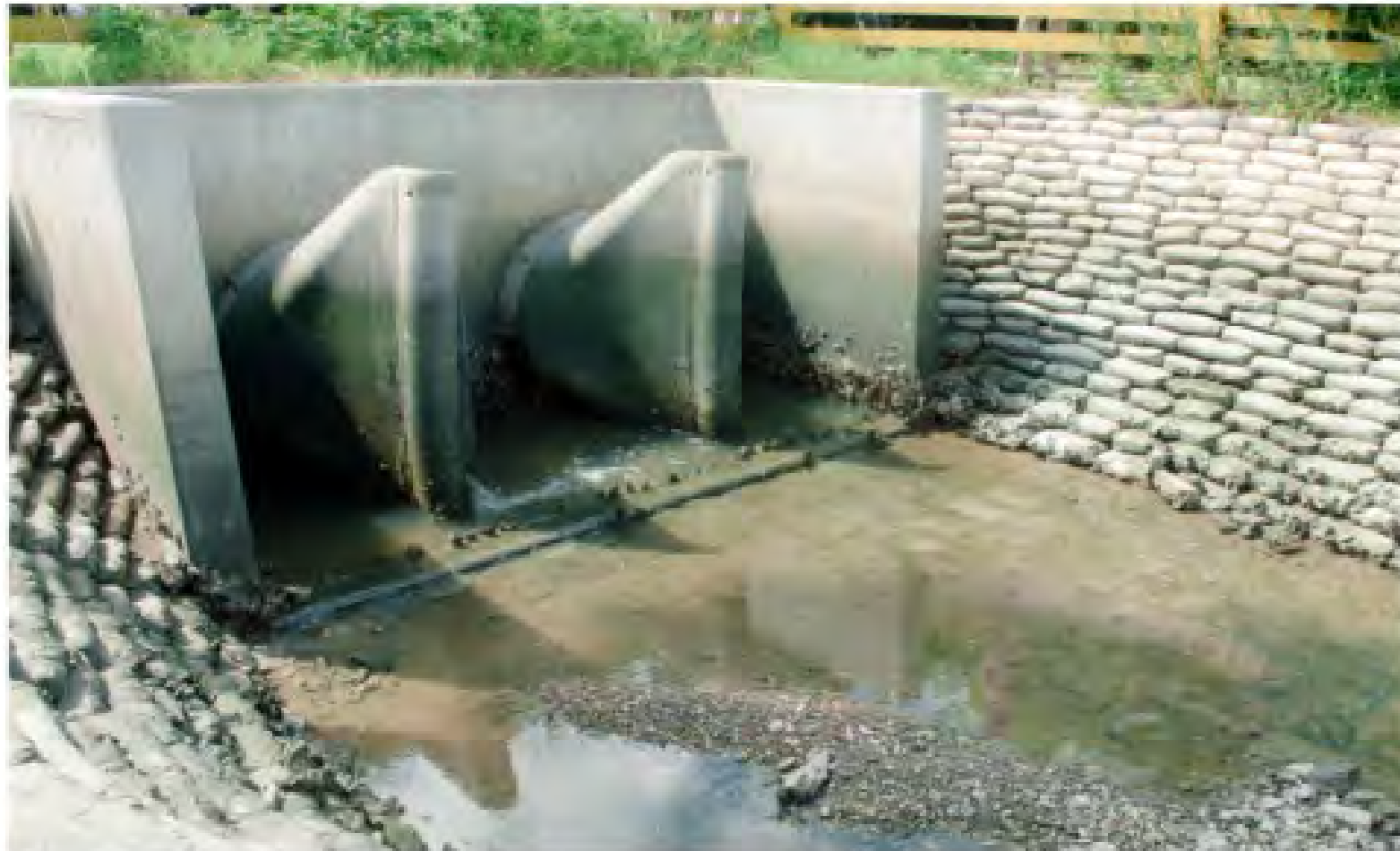
FIGURE 4.9: STORMWATER TIDAL BACKFLOW PREVENTERS, NEAR INTERSECTION OF 14 TH ST. AND VENETIAN DR.
